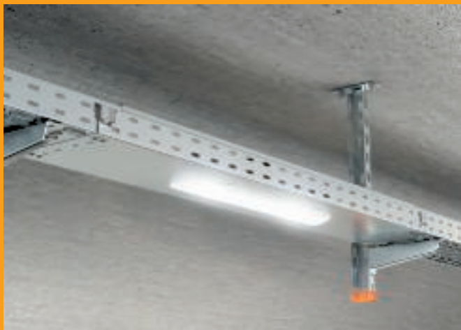
Luminaire support systems
